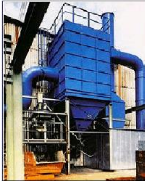
Figure 4.4 - Picture of an industrial baghouse
