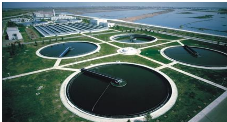
Figure 5.4 - Circular settling tanks
